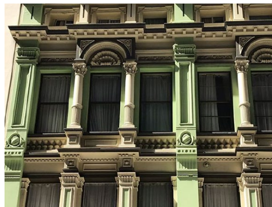
18 Detail view of moulded detailing to pilasters and columns Source: City of Sydney Council, August 2020
